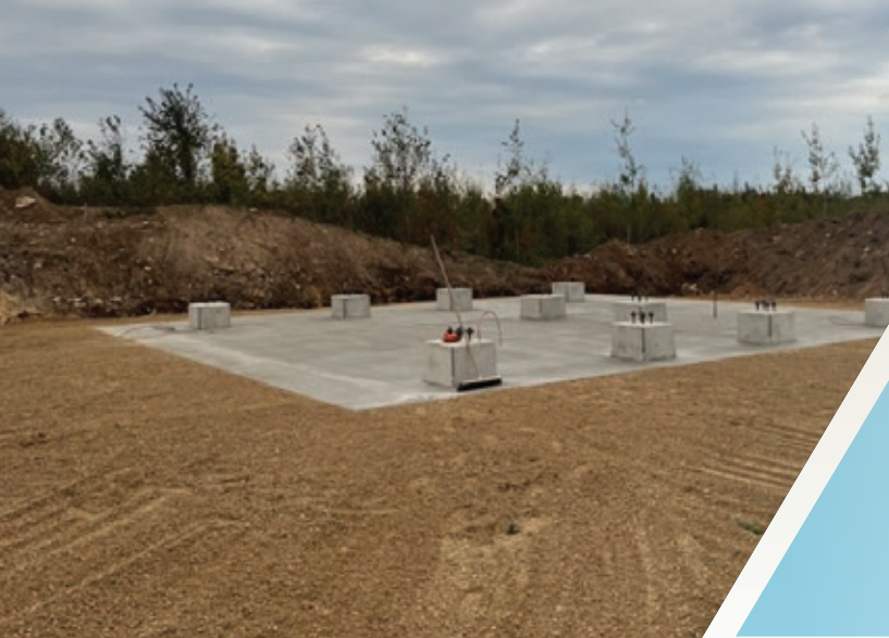
Plant infrastructure foundation installed at the Rexton site in 2025 which utilized GRAYBOND™, a low carbon cementitious solution produced by Graymont.
