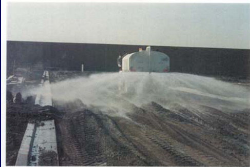
Water is a key ingredient in each stage of the lime stabilization process. Moisture is added to the lime treated soil after initial mixing and the soil is allowed to "mellow" in an uncompacted state overnight to allow for complete hydration of the lime and breakdown of the clay soil.
