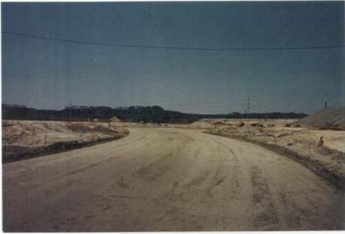
The lime treated soil after completion of final compaction with the smooth drum roller.
