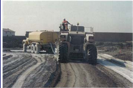
The water truck is connected to the mixer as water is pumped through the mixer and into the soil for hydration of the lime. Note the degree of mixing after only one pass of the mixer. Initial mixing consists of two passes with the CMI RS-500B.
