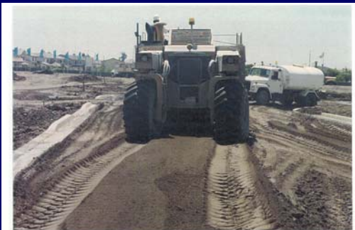
After the required mellowing period, the soil-lime mixture is remixed until gradation specifications are achieved and the material is uniform. The soil-lime mixture is moisture conditioned to achieve the specified moisture content prior to initial compaction.
