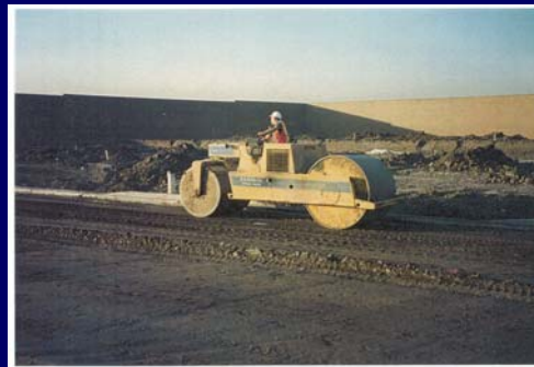
The lime treated soil is rolled with a smooth drum compactor in the "static" mode of the roller.
