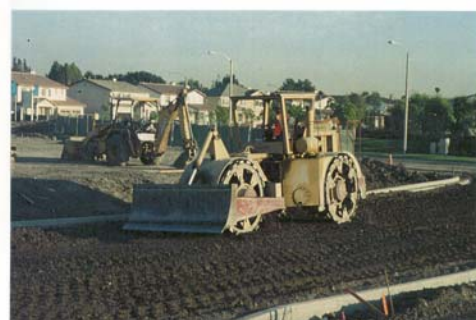
Initial compaction is achieved with a Rex self-propelled padfoot compactor. The Rex compactor has the capacity to compact 12 inches of lime treated soil in-place. Typical specifications require 90 to 95 percent relative compaction.
