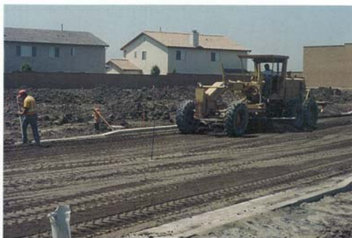
The lime treated soil is then fine graded by the paving or grading contractor to within the paving elevation tolerances.
