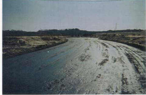
Engineers specify curing of the lime treated soil with asphalt emulsion, as seen above, or with periodic water applications - "moist cure" as seen below. Subsequent pavement layers, such as aggregate base or asphalt may now be placed over the lime treated layer.
