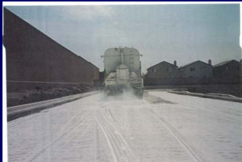
Dry lime is spread with the distribution truck at the engineer's design rate of application.
