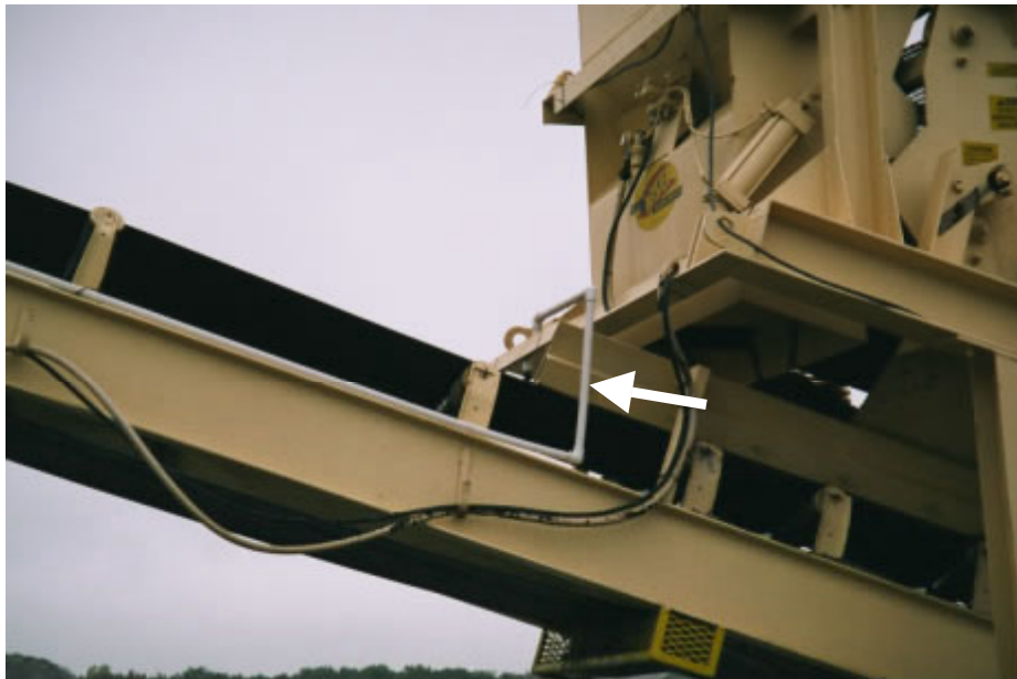
Figure 5: Water delivery system mounted over aggregate belt conveyor (see arrow)
