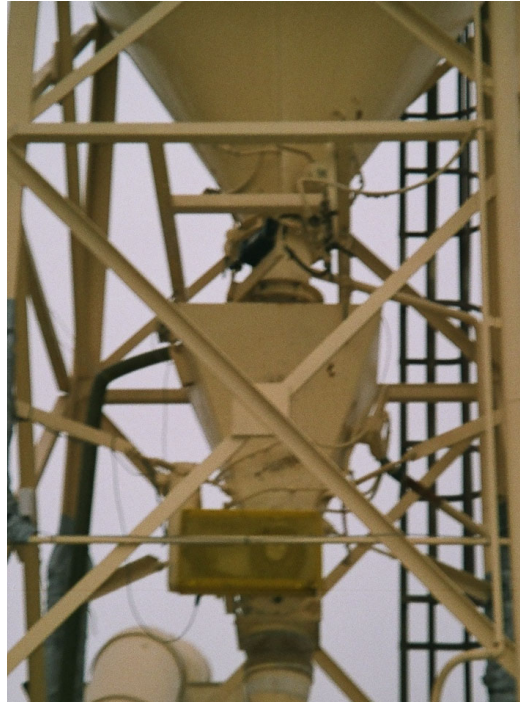
Figure 4: Hydrated lime is dispensed from the silo through a weigh pot
