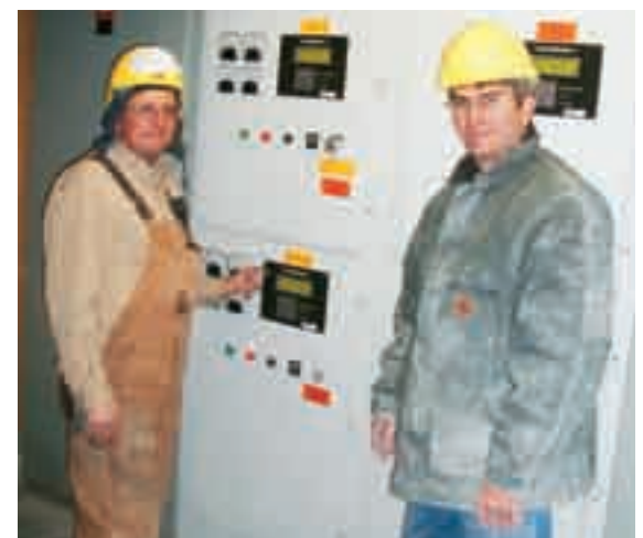
Phil Marquis (right), Superior plant manager inspects the control panel for Kiln 3's electrostatic precipitator for controlling particulate emissions from the kiln with Plant Electrician Dan Mackey.
